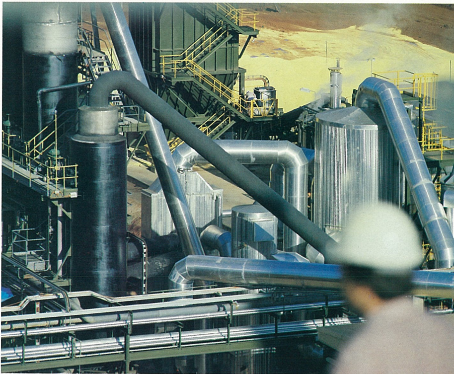
Sulphuric acid manufactured in the Plant left at Ranger is used to leach uranium out of the ore after grinding.
