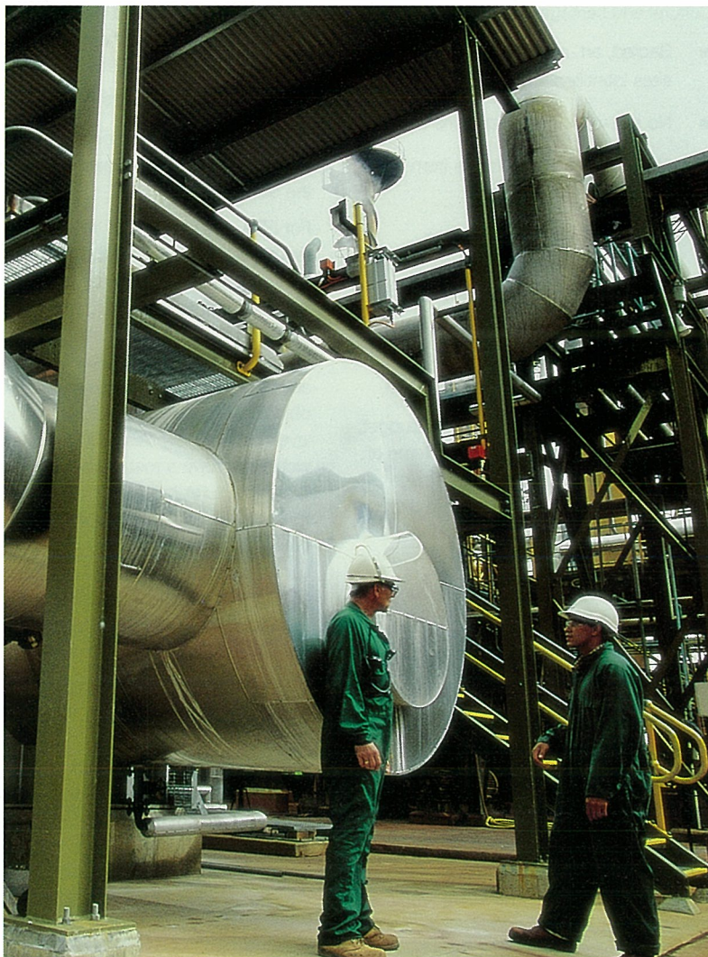
Ray Korljan (left) and Bradley Alderson, discuss the new sulfur burner and waste heat boiler at Ranger Mine.
