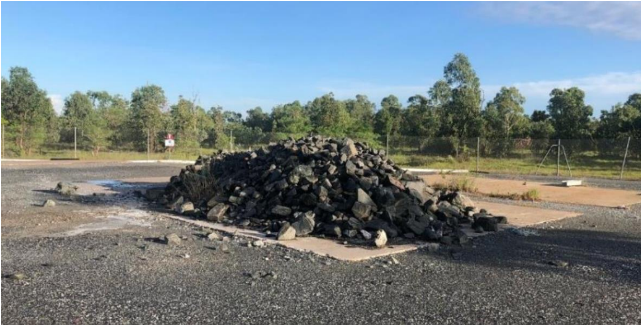
Plate 4-31: Coarse rockfill placed on top of the backfilled R3 Deeps ventilation shaft
