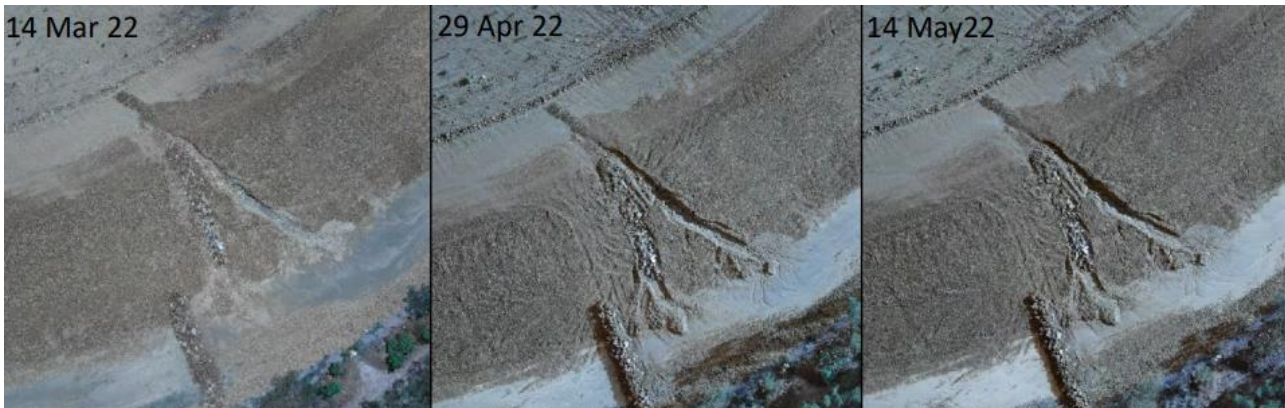
Plate 4-7: Back-cutting erosion on the steeper slope leading into the temporary perimeter drain (2022)
